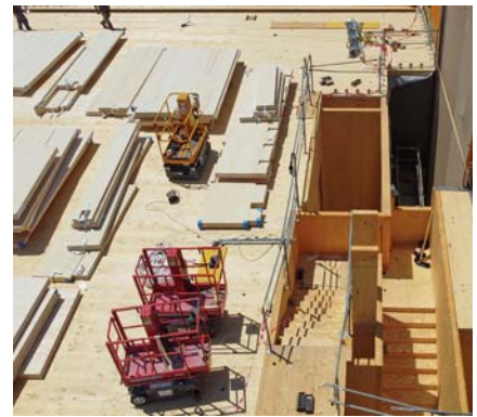
Aerial view of the assembly of the structure. CLT panels stacked on the top floor.
