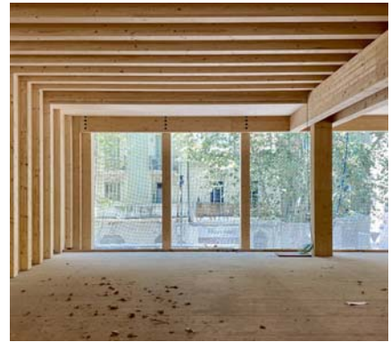
Construction process. GLT posts and beams and CLT slabs in the first floor.
