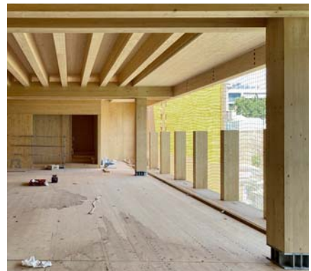
Timber structure with GLT posts and beams, CLT core in the background.
