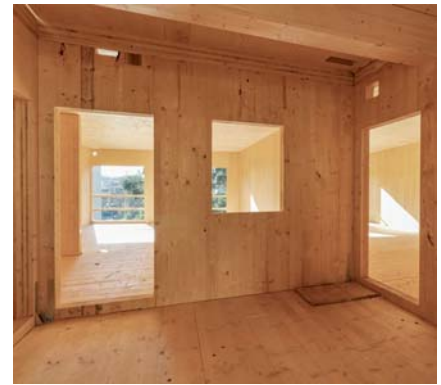
CLT interior walls Celobert cooperativa https://n9.cl/9ko3r
