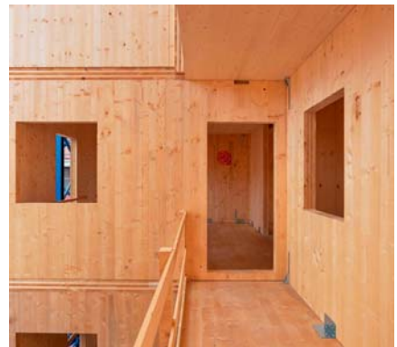
Prefabricated CLT walls with window and door openings Guifré de Peray | Celobert cooperativa
