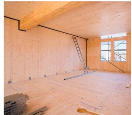
CLT panels used as floors and walls and GLT beam. Queima Films https://n9.cl/caj8l
